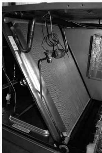
Evaporator Coil/Filter Access
