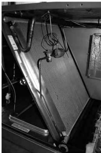
Evaporator Coil/Filter Access
