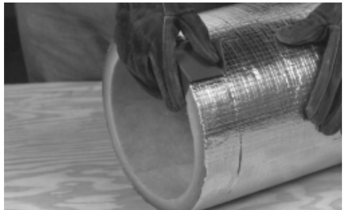
2. Using shiplap cutter to make male shiplap. Cutter is positioned to cut into exterior of duct wall.
